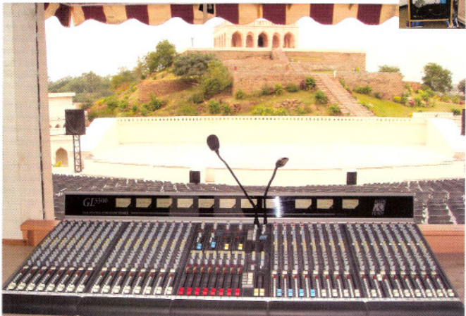
A view of the amphitheatre taken from the A/V control room at the rear end. (Inset) The rack-mounted A/V equipment in the control room
